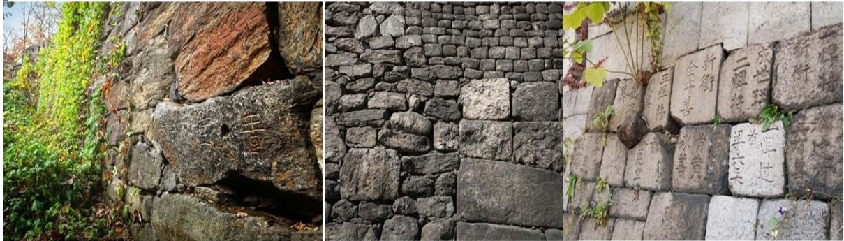
Fig1. Three major forms of wall constructed in three separate periods, Seoul Metropolitan Government
