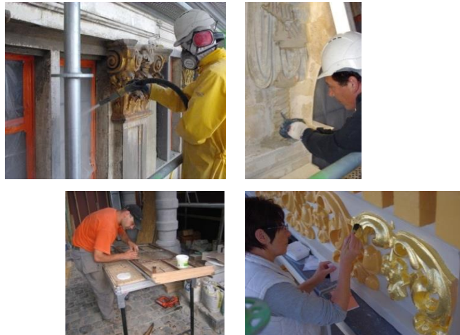
Façade cleaning, stone and windows restorations, guiding elements © Ville de Bruxelles, Département Urbanisme, Cellule Patrimoine Historique These works were made in 2003-2004 (1).
